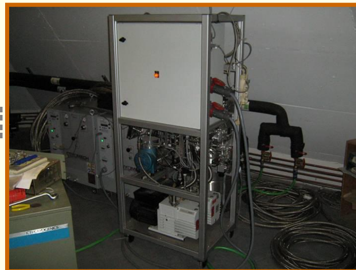
The dilution gas handling in the basement
